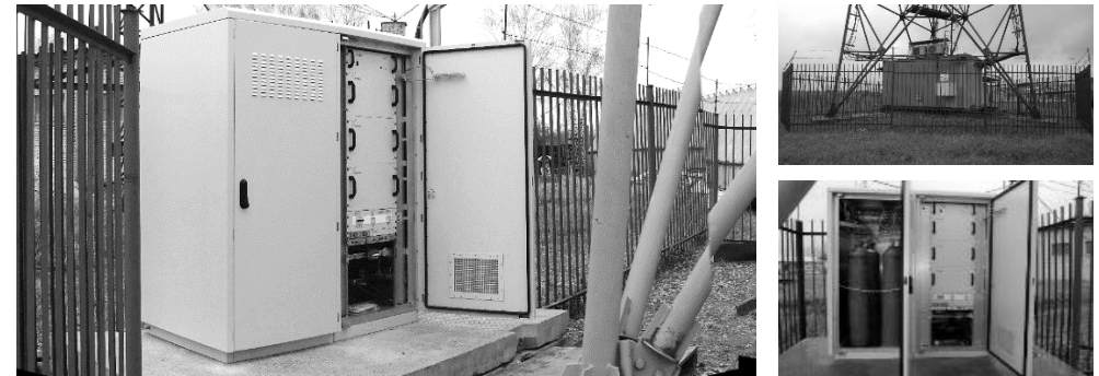
Pilot project with MTS – Base station power supply ASTRA system 7,5 kW
